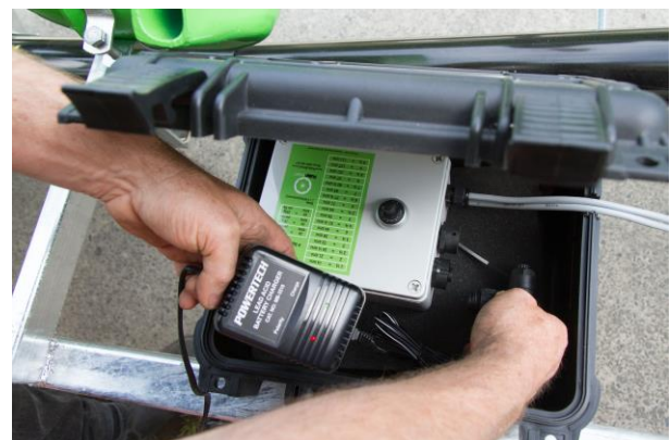
Figure 6: Plugging in charging adaptor
